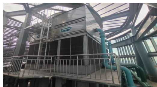
Yuexiu REIT transformed the cooling tower of Four Seasons Hotel Guangzhou. After transformation, the electricity consumption and water consumption of air conditioning decreased respectively by 21.5% and 23% compared to 2019.
