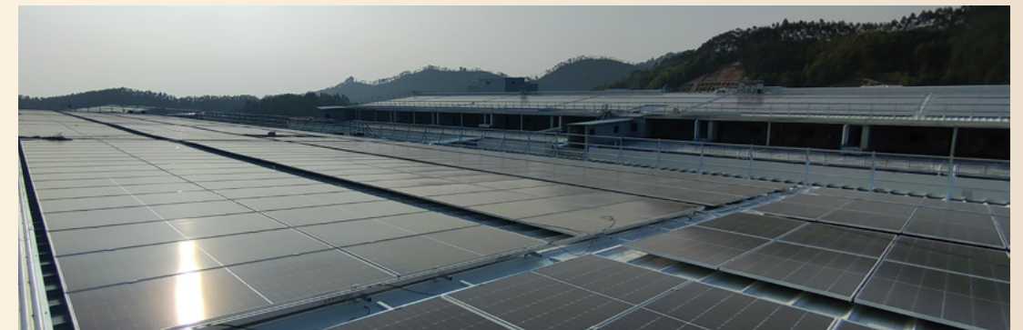
Yuexiu Capital PV Project
