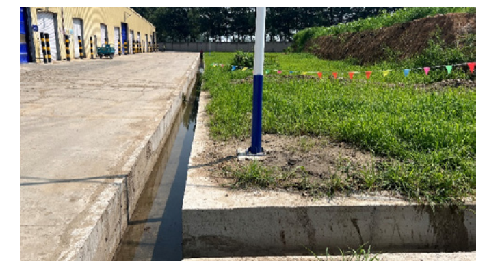
Rain-sewage diversion system of Yuexiu Huishan
